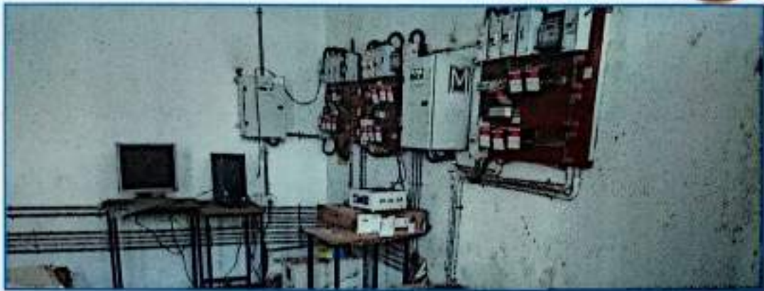
Fig. : Photovoltaic cell Control Unit
