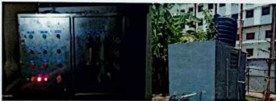
Fig. : Reverse Osmosis Water Unit
