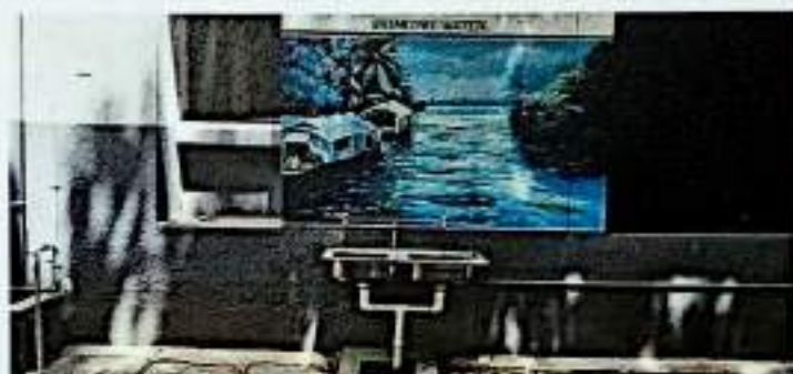
Fig. : RO Based Drinking Water Unit Installed in the campus
