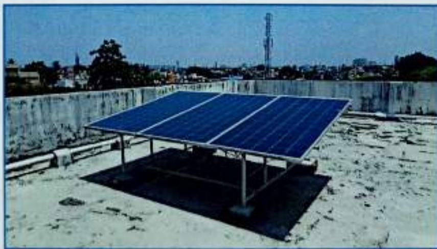
Fig. : Solar Power Plant Installed in the campus
