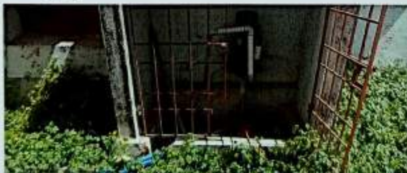
Fig : Bore wells
