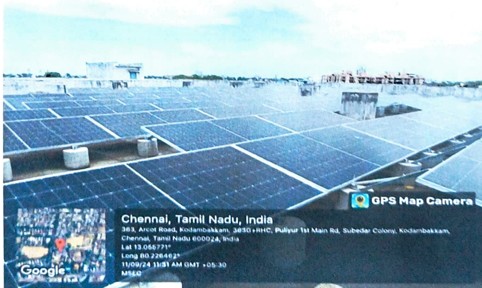
Figure 2. Installed solar panels in Main Block
