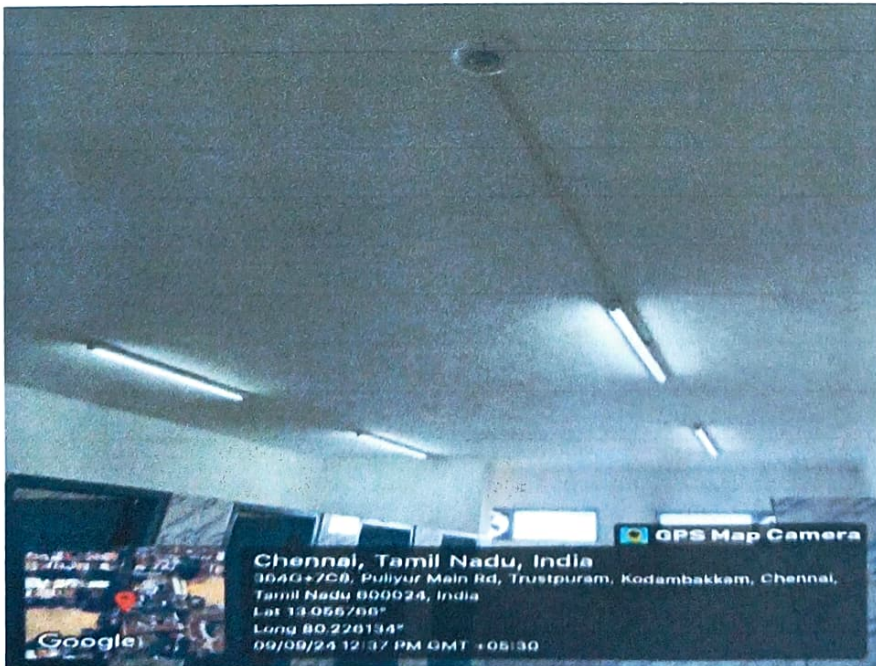
Figure 2: Installed Sensor based Lights in Restroom(Main block)
