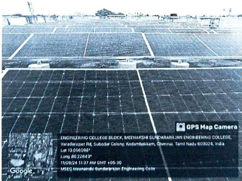
Figure 1. Installed Solar Panels in Main Block
