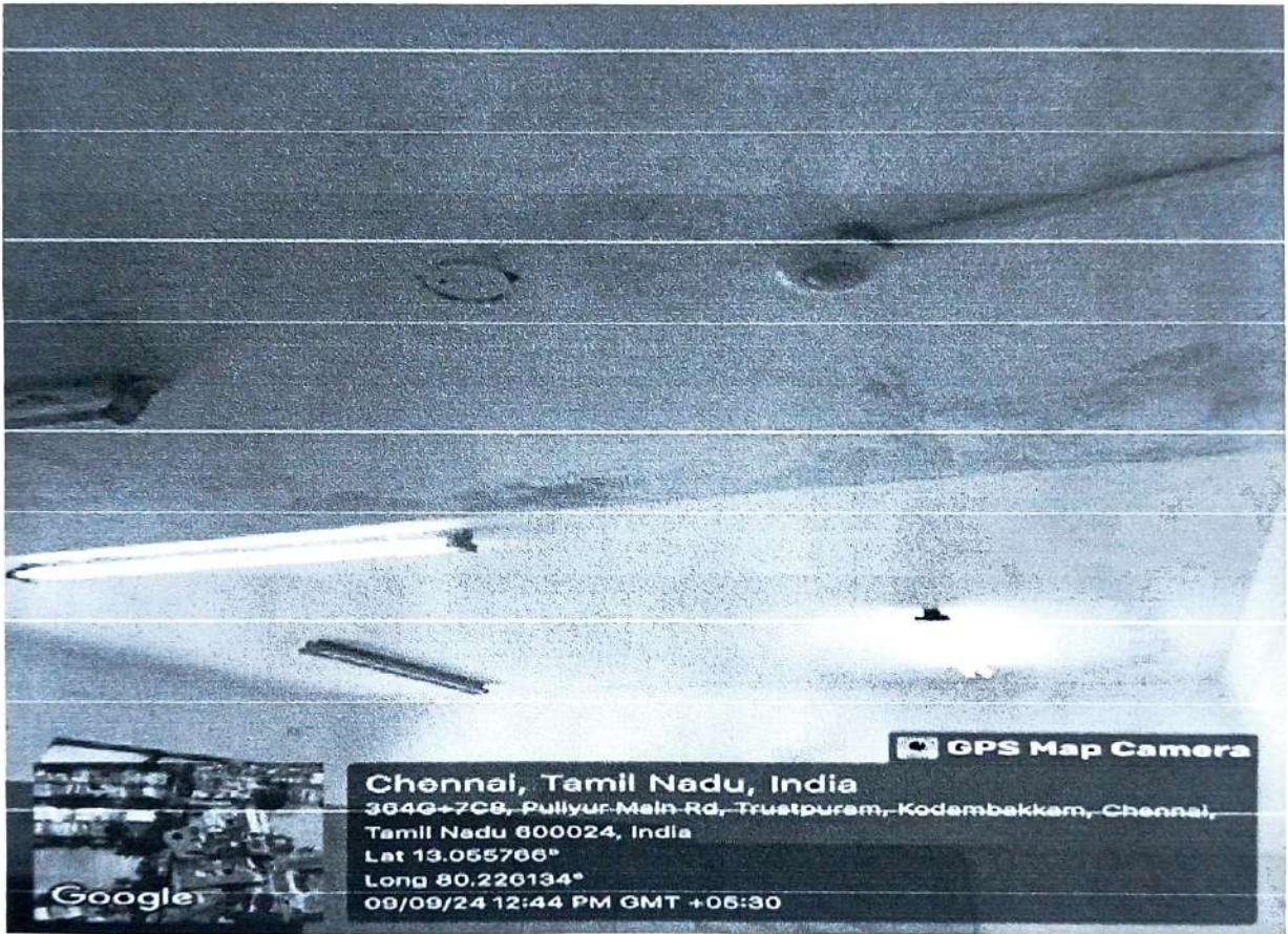
Figure5. Installed Sensor based Lights in Restrooms(Mech block)
