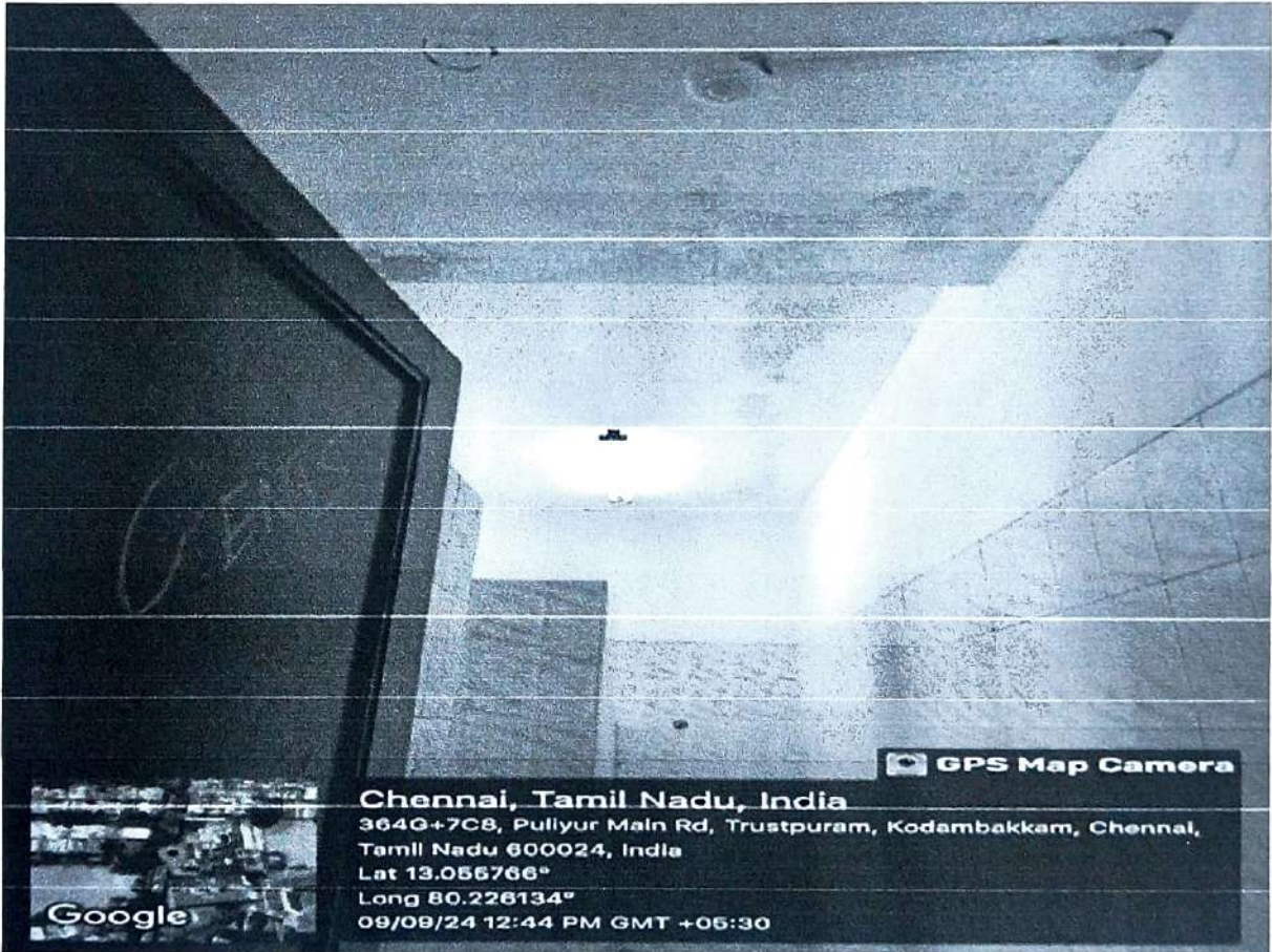
Figure 3. Installed Sensor based Lights in Restrooms(Civil block)
