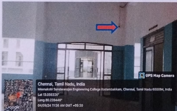
Fig. 6. : CCTV Camera at Mechanical Block Entrance
