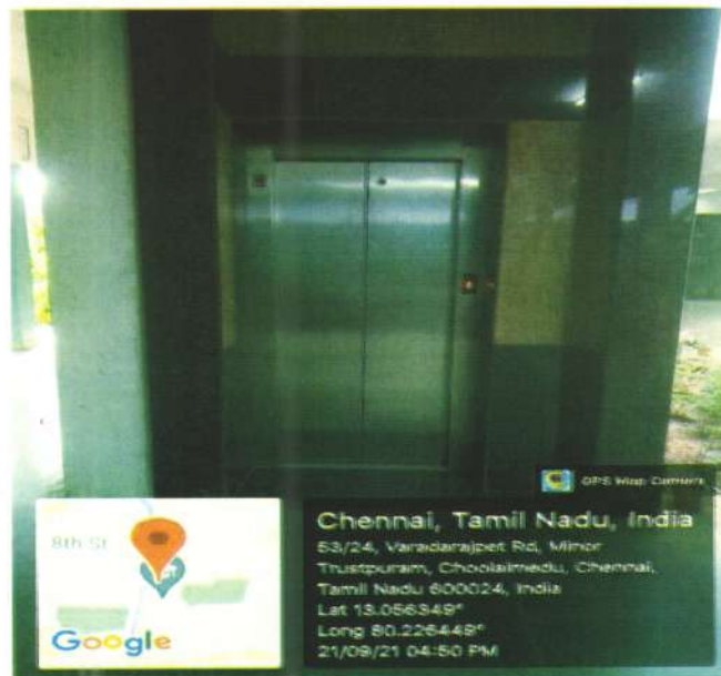
Figure 3. Lift facility in Sri Abhinav Vidhya Theertha Block (Main block )
