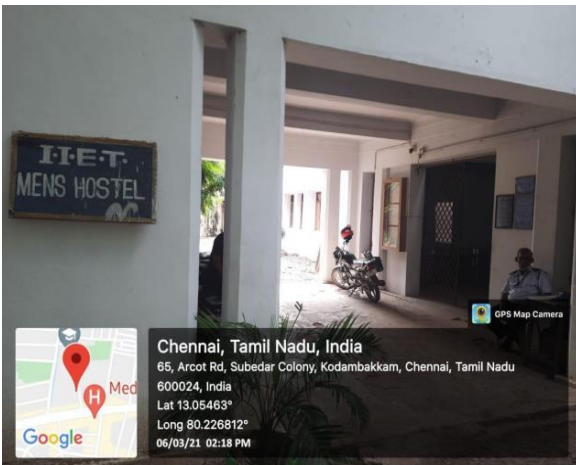
iii) CCTV Camera at Boys Hostel
