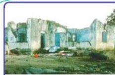
(a) Building with no horizontal lintel band: collapse of roof and walls
