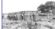
(b) A building with horizontal lintel band in Kilari village: no damage
