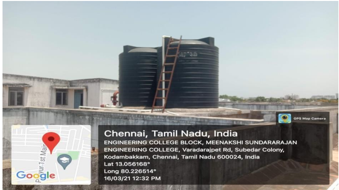
Fig. 7 : LOCATION: MECHANICAL BLOCK
