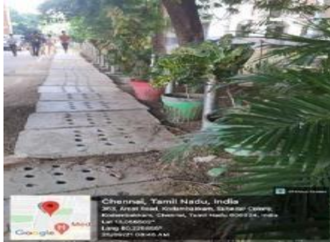
Fig. 5: Liquid waste Management: Effective rain harvesting system
