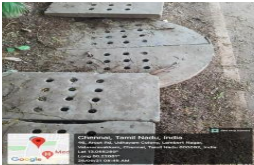
Fig. 7 : Rain Water Harvesting
