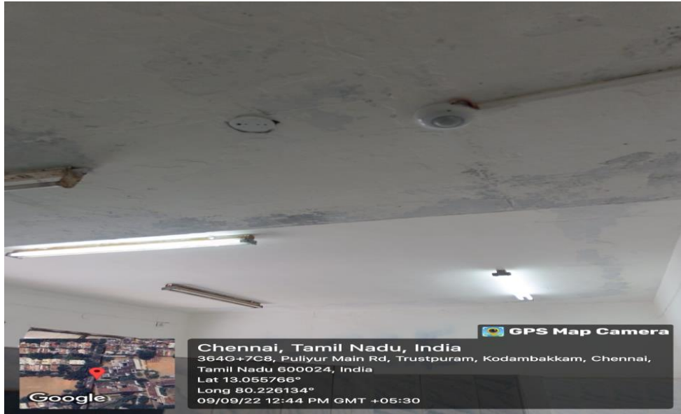
Figure5. Installed Sensor based Lights in Restrooms(Mech block)
