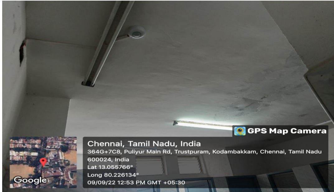
Figure 4. Installed Sensor based Lights in Restrooms(Civil block)
