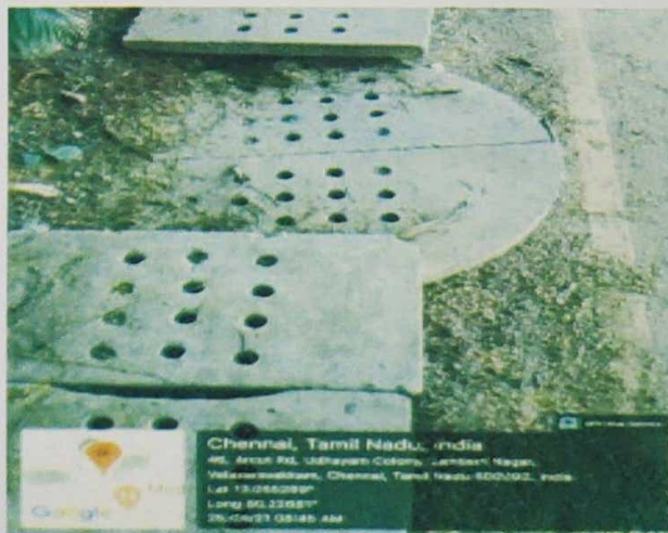
Fig. 7 : Rain Water Harvesting
