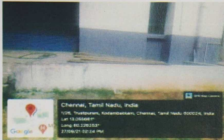
Fig. 2: Civil Block - Solid waste Management: Composting Back side
