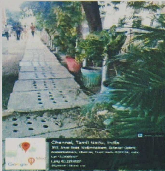
Fig. 6: Liquid waste Management: Effective rain harvesting system
