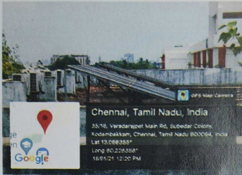
Figure 1. Installed solar panels in Sri Vidhushekhara Bharathi Block (civil block)
