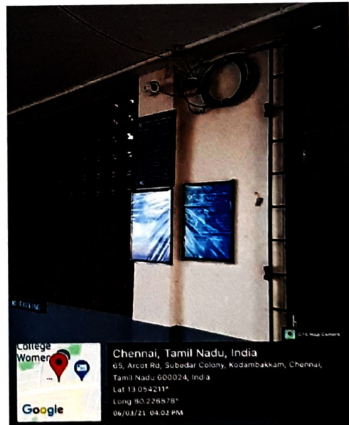
Fig. 8. : CCTV Camera at First year block
