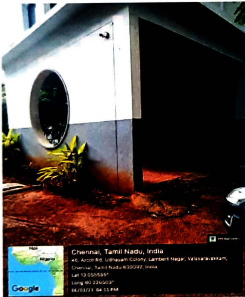
Fig. 7. : CCTV Camera near parking zone
